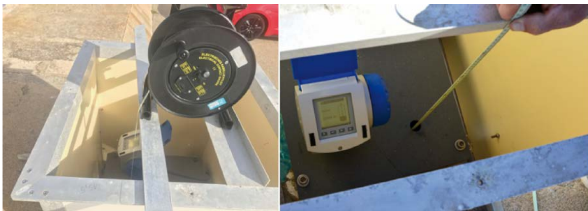
Figure 7. Control of the Ajaccio radar tide gauge using a contact probe.
