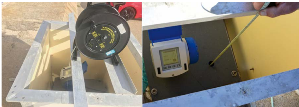
Figure 7. Control of the Ajaccio radar tide gauge using a contact probe.
