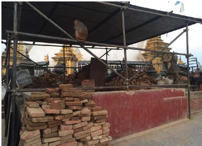
THE BASE OF THE STUPA BEFORE RESTORATION The original base of the stupa was covered with a thick layer of cement plaster and oil paint. View from the south-west. © UNESCO | D. Andolfatto | Nov 5 2017
