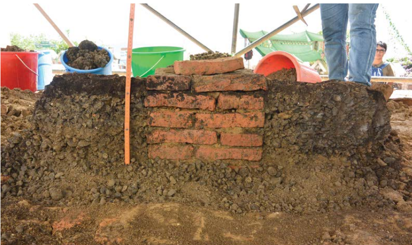
THE CENTRAL SHAFT EMBEDDED IN TSHA TSHAS View towards the north-west. © UNESCO | D. Andolfatto | Sep 16, 2016
