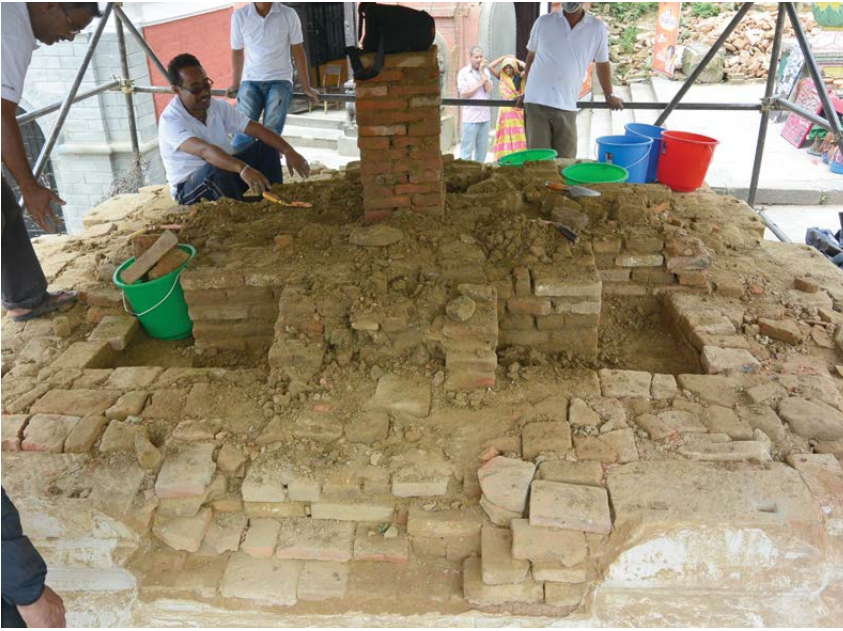
THE CENTRAL SHAFT AND L-SHAPED VOIDS View from the east © UNESCO | D. Andolfatto | Aug 29, 2016
