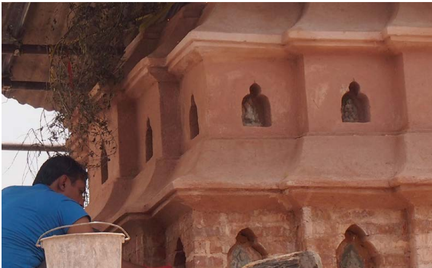
TASHI GOMANG UNDER CONSTRUCTION Application of the first coat of a lime and brick dust plaster. © UNESCO | T. Schrom | Jul 3, 2017
