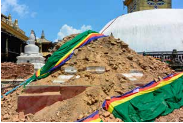
Fig 7. Tashi Gomang Stūpa shortly after its collapse. 1 st May 2015. © D. Andolfatto/UNESCO Kathmandu
