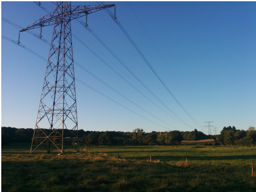
Figure 1: A common high voltage transmission line.
